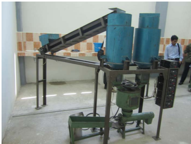
Coal blending equipment
