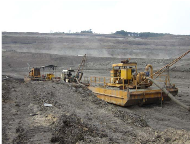
Mechanical dewatering pump
